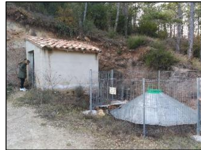
Automatic pumping of water from the natural spring
