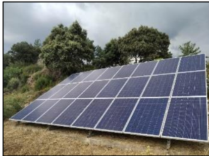
5.7 kWp of PV
