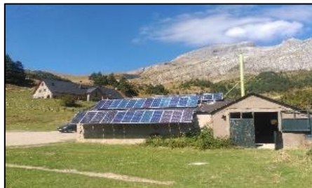
4 kWp of PV
