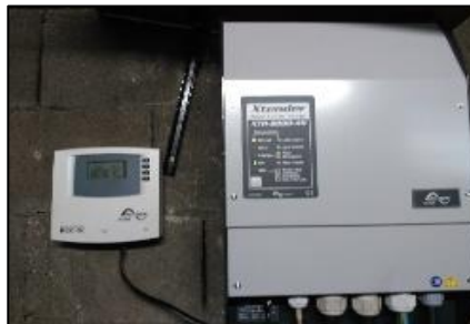
Automatic control of batteries and genset operation
