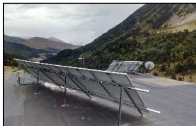
2.5 kWp of PV
